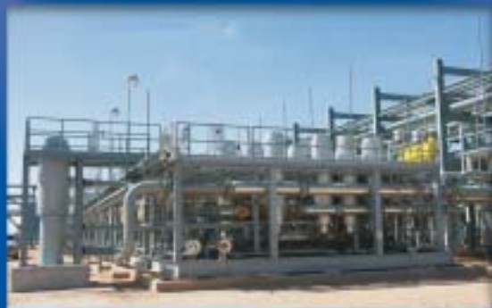
30" membrane (left) and 16" membranes (right) at NATCO's 550 MMscfd SACROC facility near Snyder, Texas
