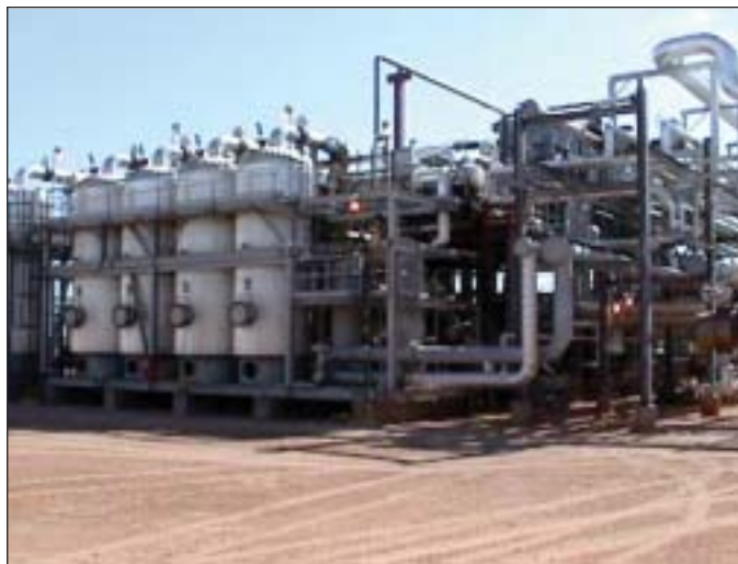
Occidental's existing dehydration unit prior to CO 2 -removal unit can treat 100 MMscfd (Fig. 8).
