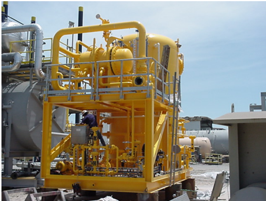
Figure 2. A 40,000 BWPD water treatment skid is shown that closely couples deoiling hydrocyclones and a vertical IGF vessel.
